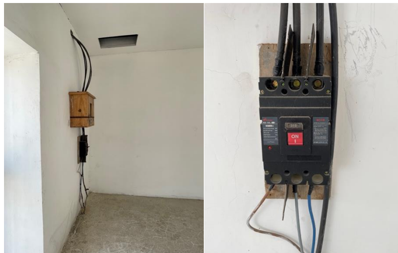
Figure 4: Covid Center Grid connection point
